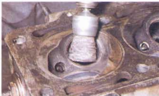
15 Using a wire brush gripped in the chuck of an electric drill, clean all traces of carbon from the combustion chambers
